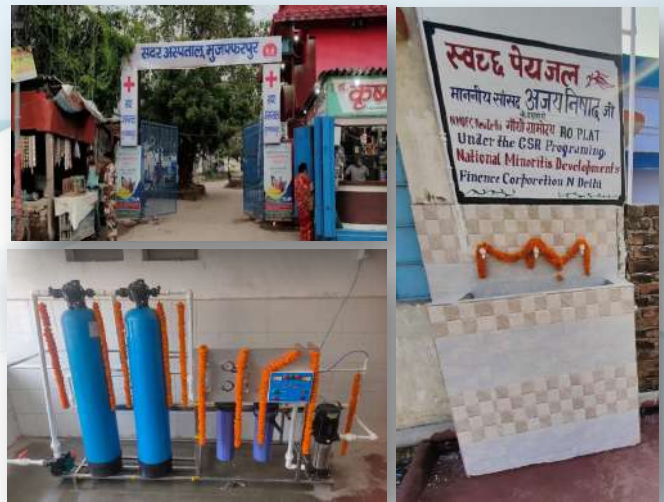
RO Plant at Sadar Hospital, Muzaffarpur, Bihar
